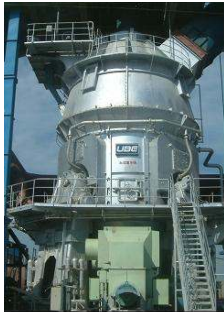
UBE Vertical Mill UM46.4SN (Made in Japan) is employed at TL's 2 nd production line
